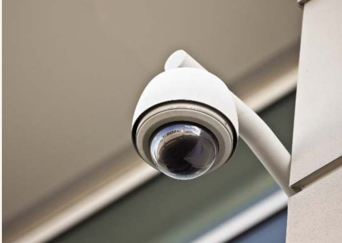
24x7 Manned Security & CCTV Surveillance
